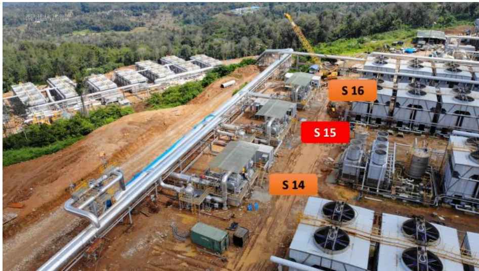
Gambar 3.13 Steam Expander Modul S-14 s.d. S-16 PLTP Sorik Marapi Unit 4 (total 39,6 MW)
