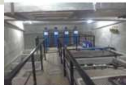
FIGURE 25. Sub Metering and Water Recycle System
