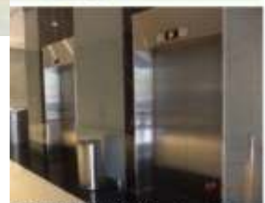
FIGURE 18. Lift/Elevator of GOP-9 Using Control Drive Microprosesor VVVF
